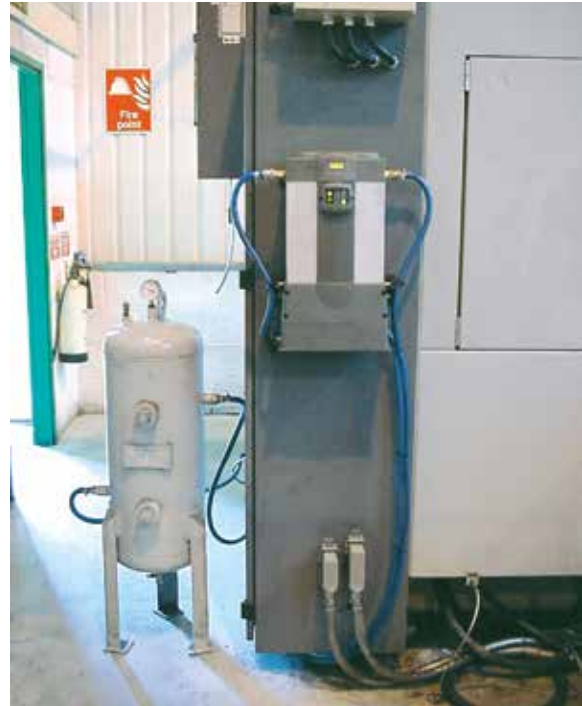
P3TJ Dry Air System installed to supply control air for a CNC machining centre
